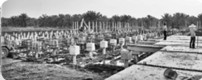
KUB Mill at Mukah - Supply of IBS hollow core slabs and square piles
