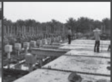
KUB Mill at Mukah - Supply of IBS hollow core slabs and square piles
