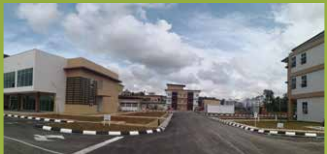
Infa Campus, Kota Samarahan, Kuching - Supply of foundation piles and IBS components
