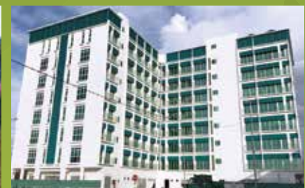
8 Storey Apartment, Bintulu -Supply of IBS precast hollow core slabs and precast beams
